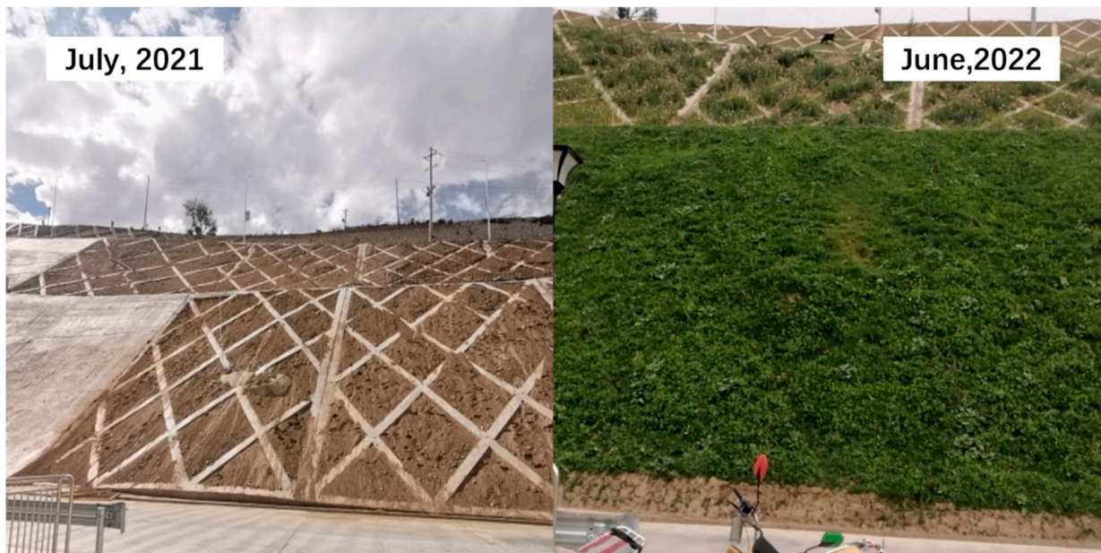
Figure 2. Comparison of restored and unrestored engineering slope at Jiacha Hydropower Station in Tibet.
