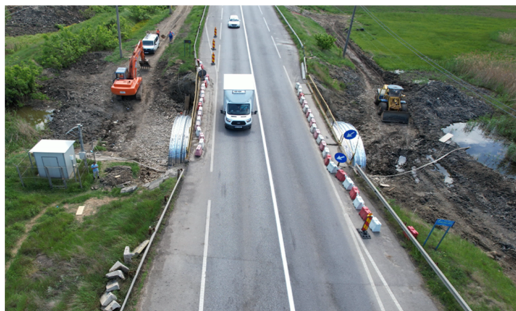
Figure 6. Aerial view highlighting the difference in width between the existing bridge and the flexible steel structure.
