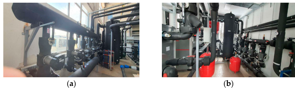
Figure 11. Thermal power plants: (a) geothermal laboratory; (b) laboratory of renewable energies.
