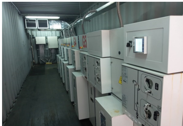
Figure 16. Control system coupling the five generators.
