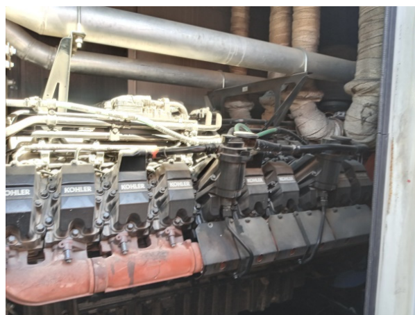
Figure 15. Main body of the larger generator.
