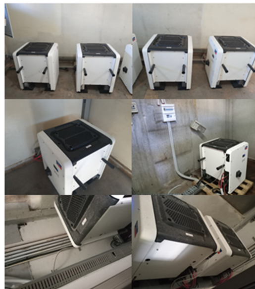
Figure 18. The installed inverters.
