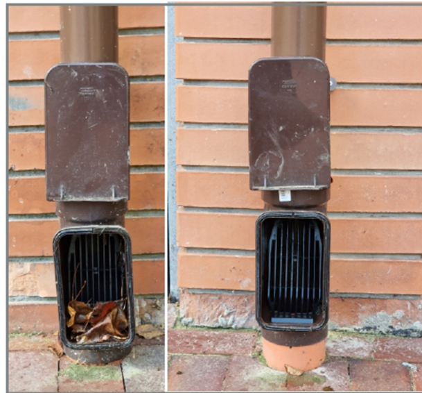
Figure 4. Photographs of cleanouts for removing dead leaves and debris from rainwater.
