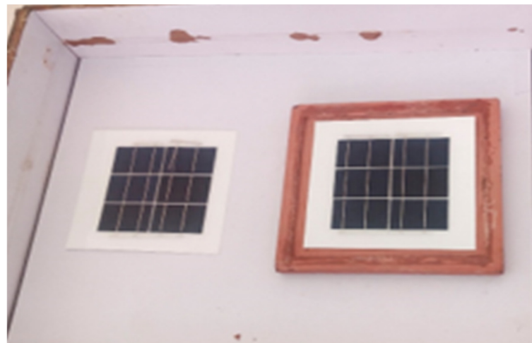
Figure 7. Normal side wall with normal solar PV and torched fly ash integrated solar PV.
