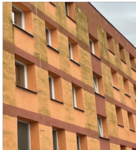
Figure 5. Significantly degraded facade of the residential housing due to biodegradation (photo: D.K.). Note: biodegradation—a consequence of the inhomogeneity of the original external wall based on lightweight based on slag concrete, construction and physical connections (on the external wall, there is no surface biodegradation, and under the windows, there is a radiator for heating in the interior, see Appendix D).
