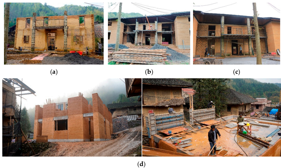
Figure 8. Water resistance performance of rammed earth walls with and without the addition of cement in a harsh construction environment and in high humidity and light rain. (a) shows the preserved existing rammed earth wall at the beginning of construction; (b) shows the collapse of an area of retained traditional rammed earth wall due to sudden rainfall during construction; (c) shows the re-mixing of collapsed earth wall materials and re-laying of masonry in the form of adobe bricks in the collapsed position, connecting the new rammed earth wall with the retained rammed earth wall; (d) shows the relatively high resistance performance of the new rammed earth wall in the face of a wet and watery construction environment.
