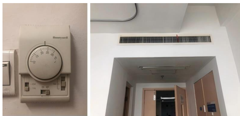
Figure 3. Photo of the primary air fan-coil system in Ningbo case study maternity hospital.
