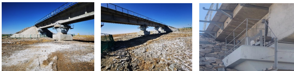
Figure 1. K1013 + 358 grid station overview.
