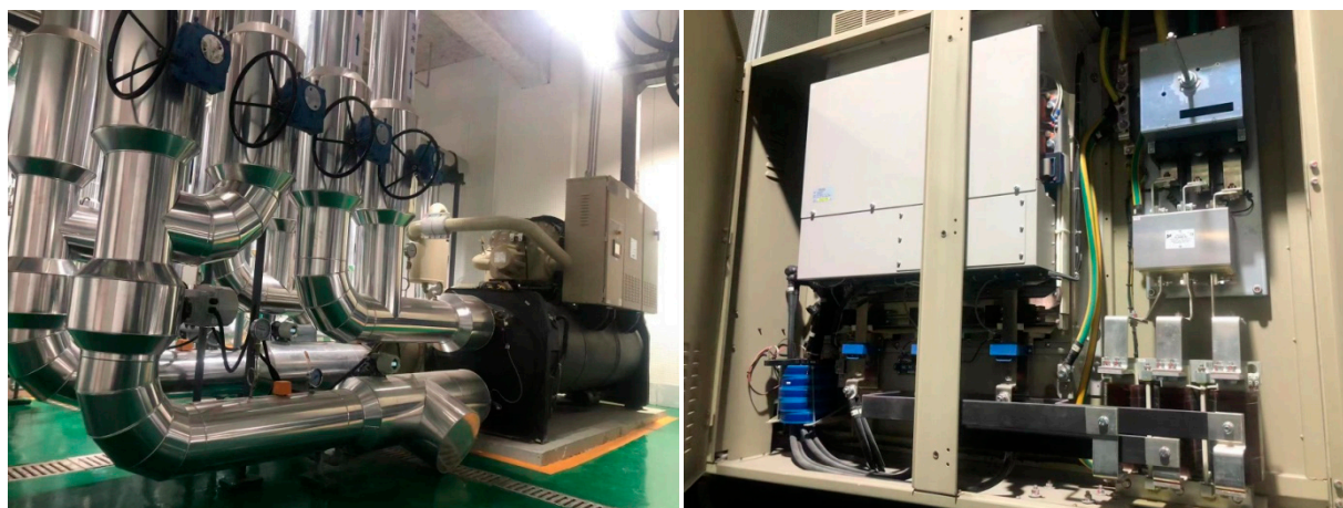
Figure 2. The heatpump heating retrofit project located in Shanxi, China.
