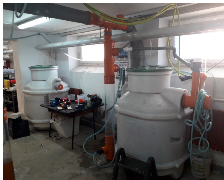
Figure 2. Septic tank of pre-treated wastewater utilized for research.
