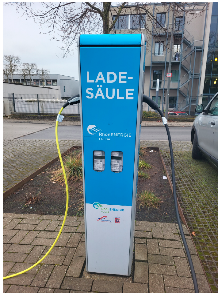
Figure 9. Example of a charging point in Germany.
