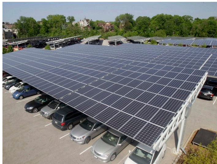
Figure 2. Parking covered with PV solar panels [7].
