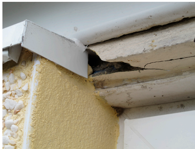
Figure 10. Damage to window head during the installation of EWI.
