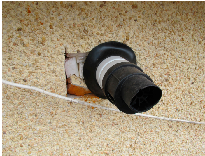
Figure 11. Poor timetabling resulted in damaged EWI.
