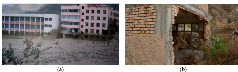
Figure 1. Damages caused by debris flow: (a) Debris flow in Zhouqu County; (b) a masonry wall destroyed by debris flow.
