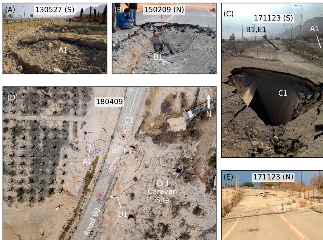
Figure 8. Road 90 sinkholes near En Gedi. Picture dates are labeled YYMMDD with look direction in brackets. For relative location, see panel (D). (A) Sinkholes west of the road (A1), after being filled with gravel; (B) Exposure of the geosynthetic sheet above a 5 m wide, 9 m deep cavity (B1); (C) sinkhole collapse on the road (C1), after almost five years of InSAR-detected subsidence; (D) Drone photo of the subsidence area. Note the circular cracks (D1) surrounding the subsidence center (E1). Blue circles mark sinkholes along the road margins and red circles mark sinkholes collapsed along the road; (E) Compressional deformation on road asphalt at the center of the subsiding area (E1).
