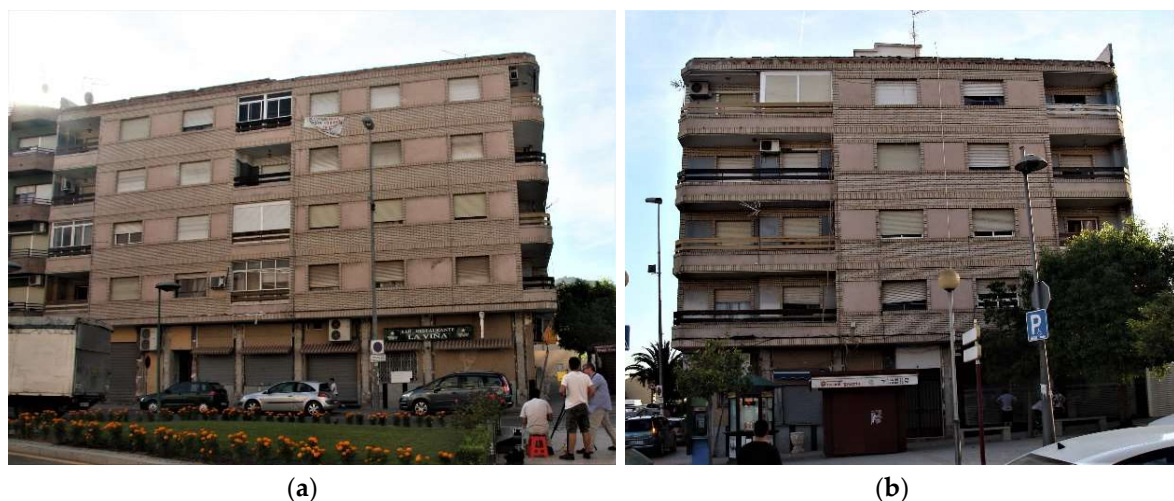
Figure 2. Main façades of the “La Viña” building: (a) longitudinal orientation, L; (b) transversal orientation, T.
