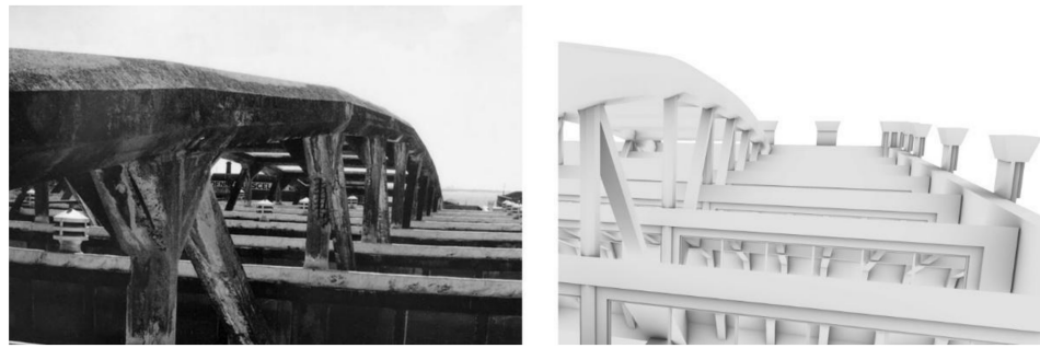
Figure 2. Left: the photo of the bow truss structure above the saw-tooth roof system. Right: the digital reconstructed model of the bow truss roof is modeled based on the reference of the previous photo.
