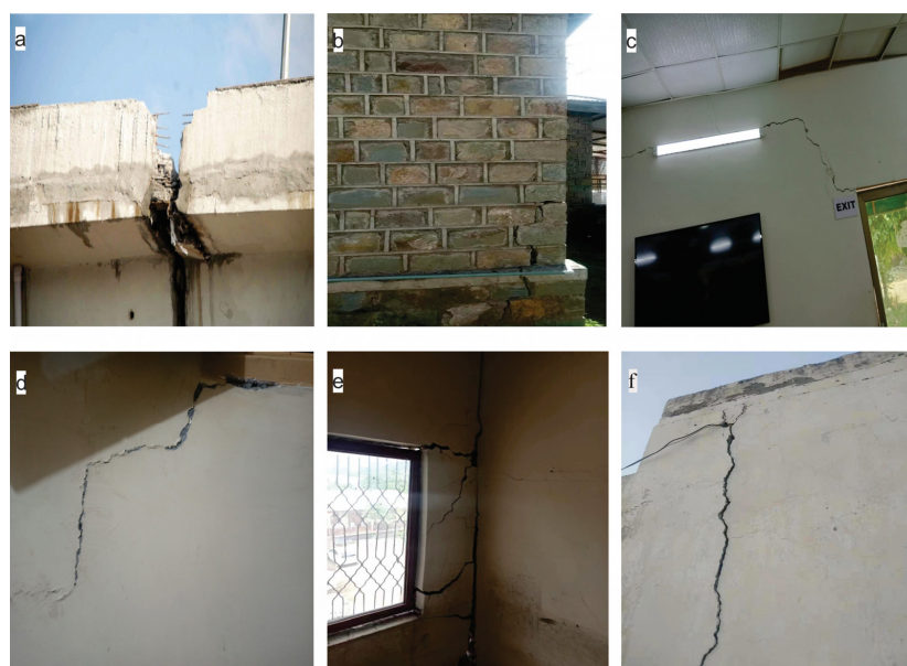
Figure 17. Cracks in the walls of different buildings within the research area. (a) Cracks in the pillars of metro track at Committee Chowk, (b–f) Cracks in walls of local houses in Raja Bazar, Waris Khan, Rehmanabad, and Sadiqabad areas.
