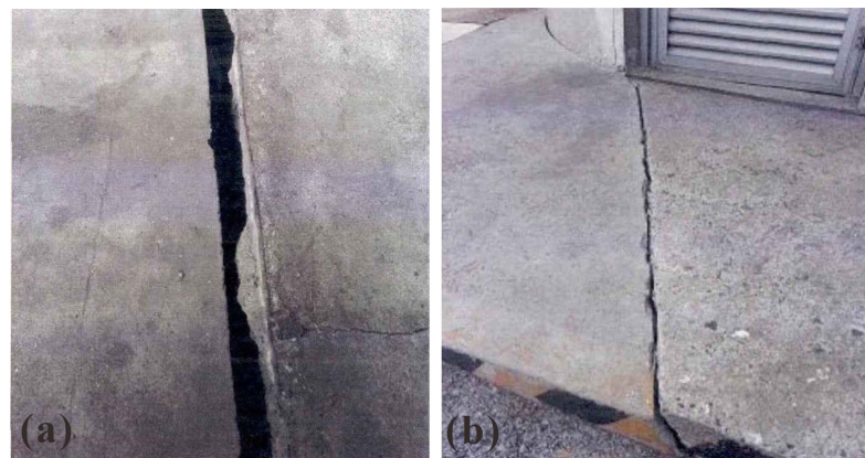
Figure 8. Ground fractures from ground deformation, (a) cracks on the transition zone in front of Terminal 1; (b) crack at the boarding bridge of Terminal 2.
