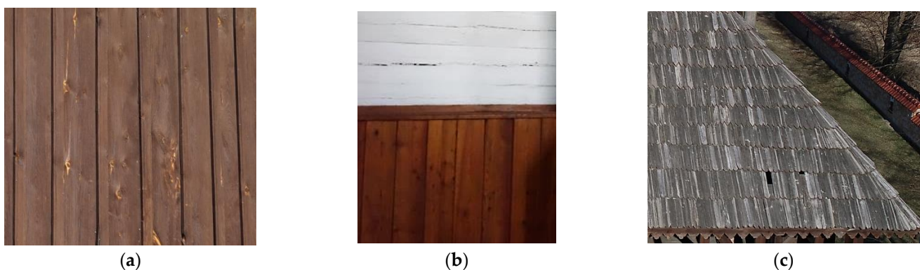
Figure 8. Identification of objects on photos: (a) formwork material, (b) walls, (c) architectural details roof with a crack.
