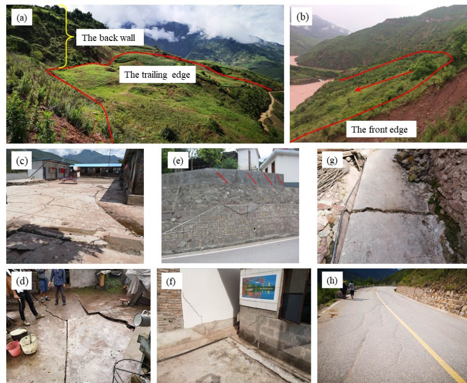
Figure 10. Field survey photos. (a) The trailing edge has sunk. (b) The front edge has slid. (c) Cracks in the Cheyiping primary school. (d) Cracks in villagers’ homes. (e) Fissures in the walls. (f) Cracks in houses. (g) Cracks in the road in the village. (h) Deformation of Bao–Tibet highway.
