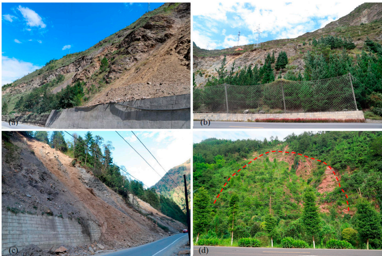
Figure 2. Mass movement events along the National Highway 318: (a–d) Disasters that distributed in different areas of the road. The red dotted line is the boundary of the disaster.
