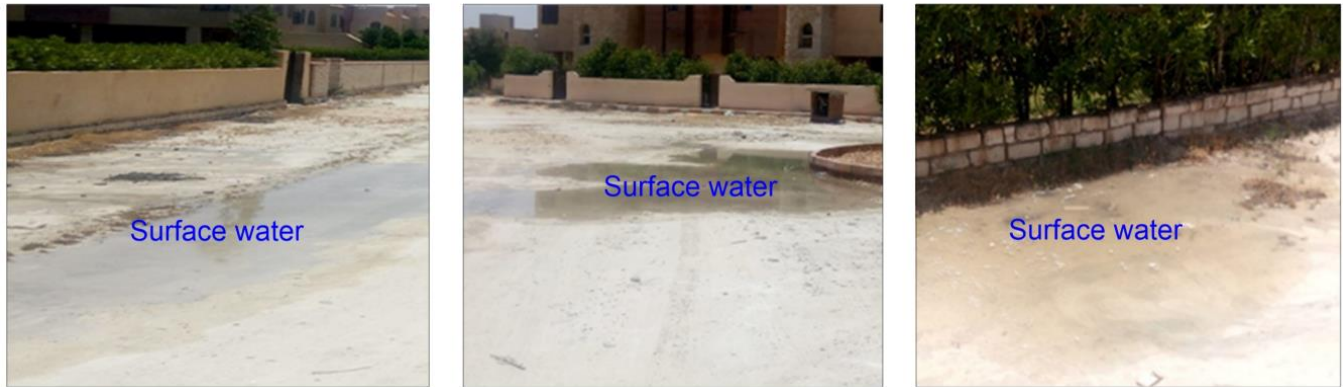
Figure 2. Presence of water leaks on certain surface areas.
