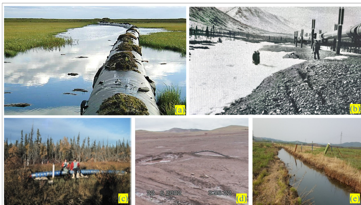
Figure 1. Common oil and gas pipeline damages in permafrost regions. (a). The Medveje gas pipeline that once was buried and now is floating in a marsh, resulting partly from the thawing of the permafrost [19]; (b). Differential settlement of the workpad in an elevated pipeline segment of the Alaska pipeline [11]; (c). Frost heaving of the buried Norman Wells Pipeline in September 1997 [20]; (d). Frost heaving and deformation at Wuli of the Product Pipeline from Golmud to Lhasa in June 2002 [20]; (e). Surface subsidence occurs in some areas where the CRCOP crosses permafrost regions, resulting in the formation of ponds.
