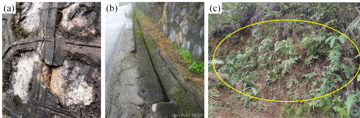
Figure 3. On-site findings in November 2018: (a) cracking of retaining wall, (b) guttering deformation, and (c) collapse.
