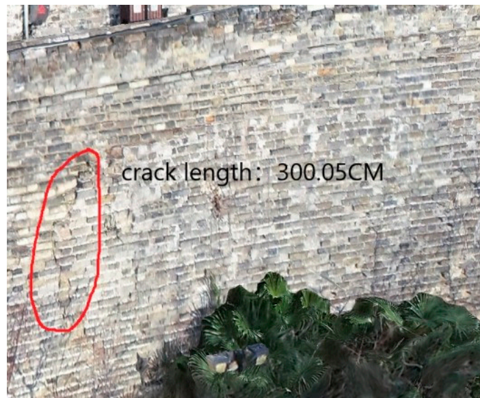
Figure 17. The longest crack in inner wall.
