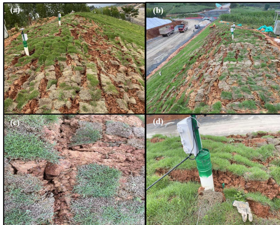
Figure 4. Shallow instability characteristics of Ningming expansive soil. (a–d) The visible cracks near the monitoring station.
