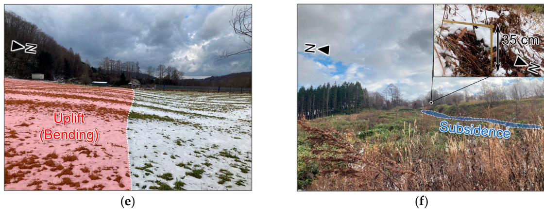
Figure 13. Ground movements on field survey: (a) cliff within Kounai-2 body; (b) cliff at the toe of Kounai-2; (c) crack at Osaru River basin; (d) tilted a catchment well at the toe of Kounai-1; (e) bending of the terrace between Kounai-1 and Kounai-2; and (f) cliffs near the western side of the main cliff of Kounai-2. The locations are shown in Figure 11.
