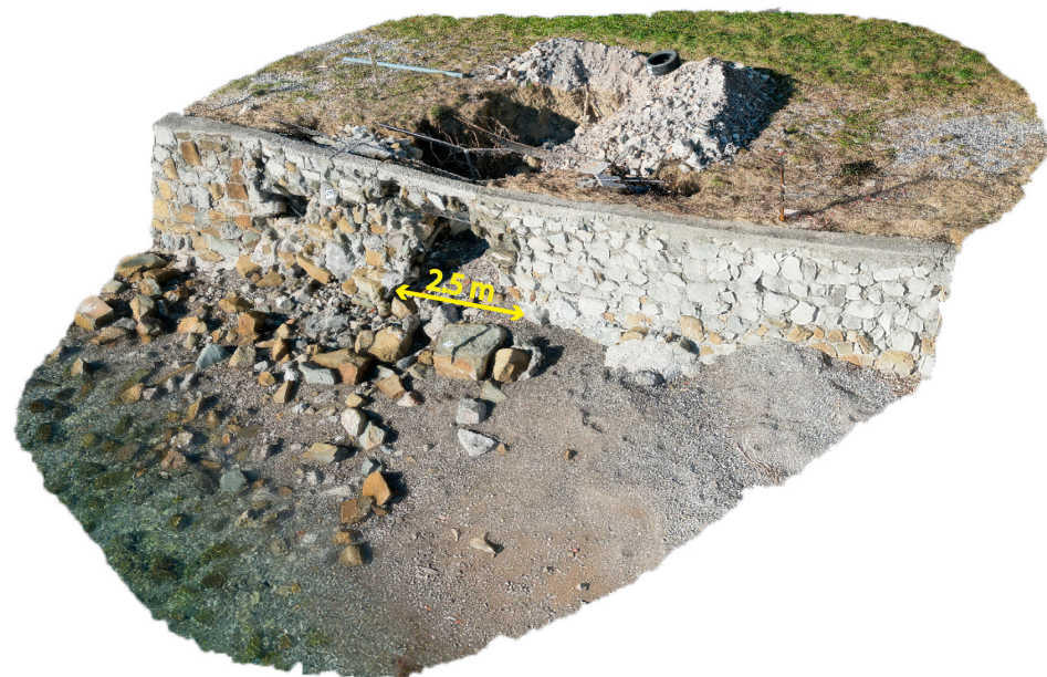
Figure 11. Three-dimension model of the sinkhole H on 29 November 2023 ( https://skfb.ly/p7Uzu , accessed on 21 August 2024). It was already partially filled with landfill material. The retaining wall is almost completely broken. View towards the north-west. The ground resolution of the model (provided by the Agisoft Metashape report) is equal to 3.34 mm/pix.
