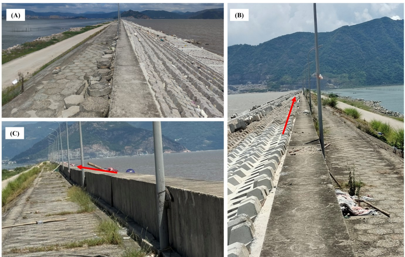
Figure 13. On-site photographs of the reclamation embankment (A). The red arrows in (B,C) indicate the occurrence of tilting and settlement of the embankment, respectively.
