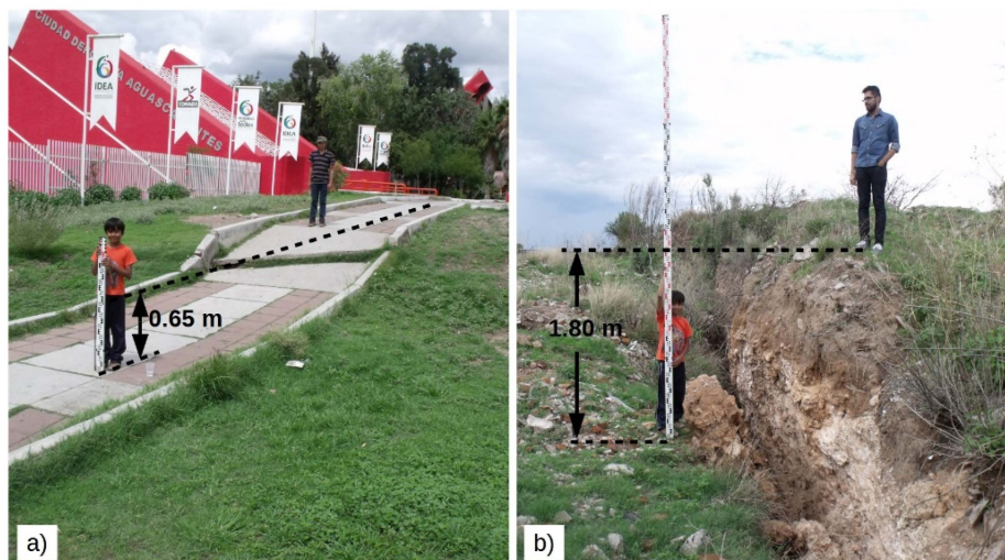
Figure 1. Surface faults due to differential subsidence in Aguascalientes. (a) Surface fault affecting man-made structures; (b) Surface faulting has developed escarpments up to 1.80 m high. The location of the subsidence-related surface faults is shown in Figure 2b.
