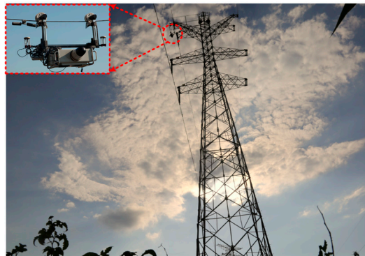
Figure 20. Photo of the tower and power lines.
