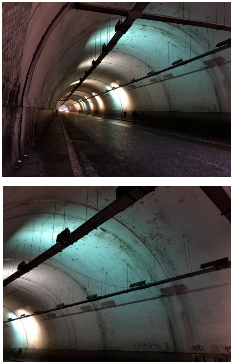
Figure 50. Photographs showing the status of the Umberto I Tunnel in Rome nearly 11 years after the renovation. Photographs taken 4 March 2018 at 17:00 (Copyright by N. Serpone).
