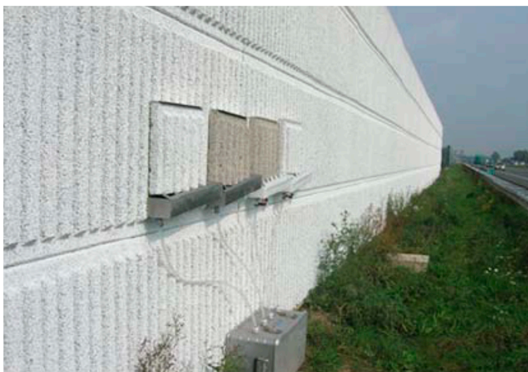
Figure 51. Example of a \text{TiO}_2 -coated concrete noise barrier erected along the A1 and A28 highways in Terschuur and Putten, the Netherlands. Reproduced from Ref. [152].
