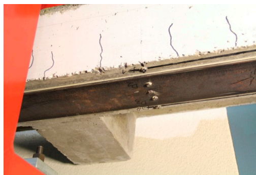
Figure 17. Bottom side of the beam in the year 2015. Surface corrosion is visible on the steel plate.
