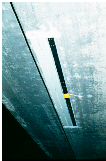
Figure 7. Applied CFRP strips on the Ibach bridge in the year 1991 (two strips were painted for aesthetic reasons).
