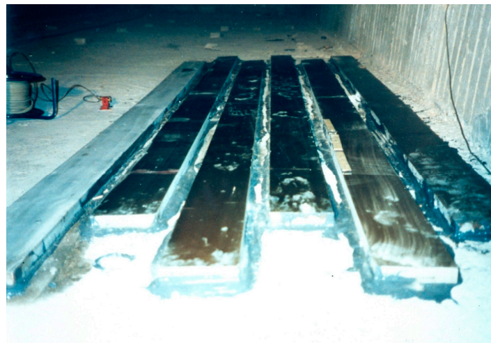
Figure 5. Glass fiber reinforced polymer (GFRP) Plates at the bottom slab of Kattenbusch Bridge (Source: Prof. Ferdinand S. Rostásy).
