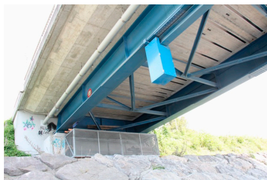
Figure 22. Underside of the bridge. The CFRP strips for the strengthening of the cross-direction are visible between the steel girders.
