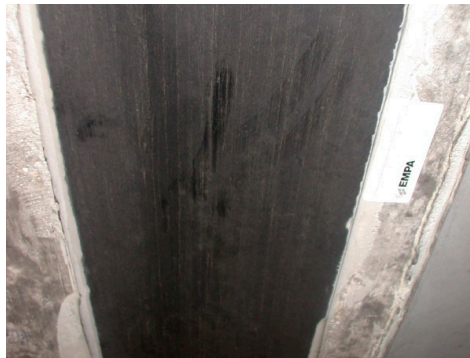
Figure 9. The photo shows the very good condition of one of the CFRP strips in the year 2008 (dust on the surface is visible).
