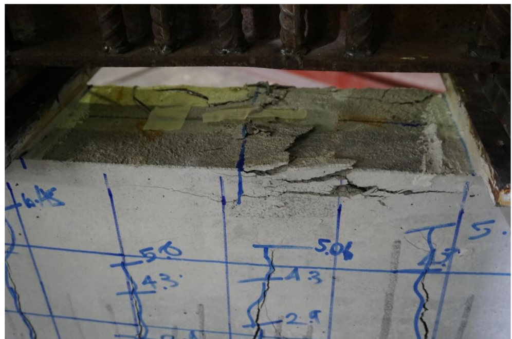
Figure 12. Typical crushing of concrete in all specimens.
