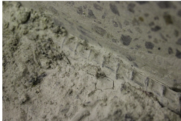
Figure 11. Steel–concrete interface on the OPC beam, showing cracks along the ribs and crushed concrete between ribs.
