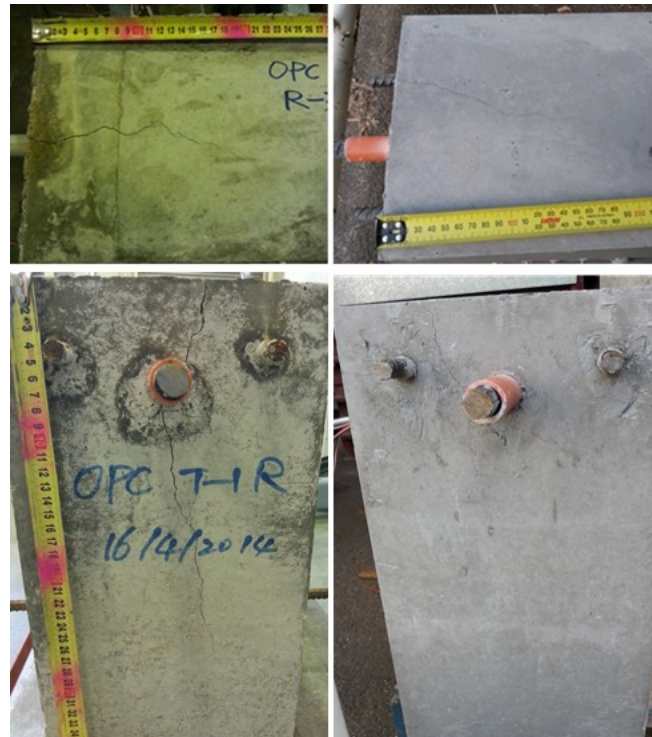
Figure 9. Comparison of the crack widths of OPC B-4 (left) and GPC B-6 (right).
