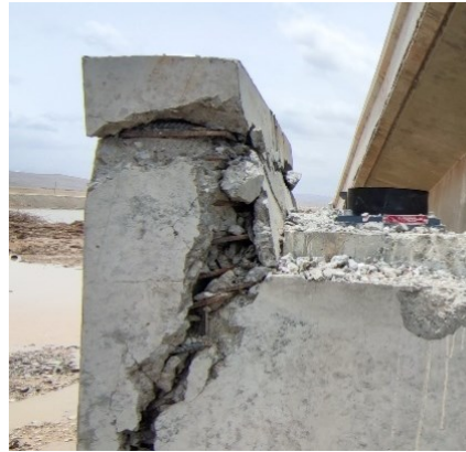
Figure 10. Seismic damage of blocks.
