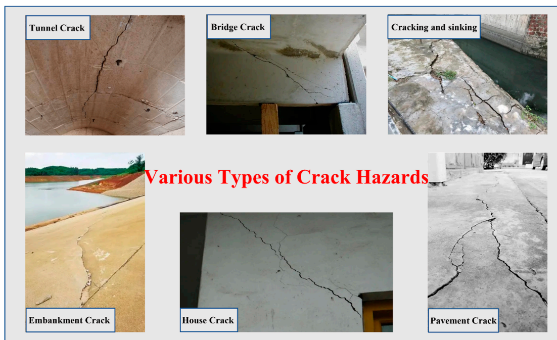
Figure 1. Several typical forms of crack damage in cement-based materials structures.
