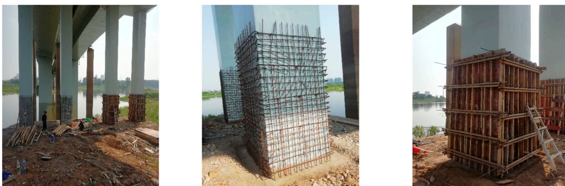
Figure 8. The preparation of high-strength, ultrahigh-performance concrete incorporating highly refined interconnected internal curing aggregates for application in the abrasion-resistant protection of bridge piers.
