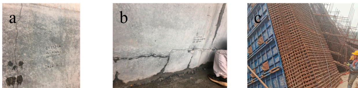
Figure 2. High-strength large-volume marine concrete presents challenges in the installation of water pipes and exhibits evidence of cracking: (a) Vertical cracking of concrete; (b) Horizontal cracking of concrete; (c) Inconvenience in the installation of cooling water pipes.
