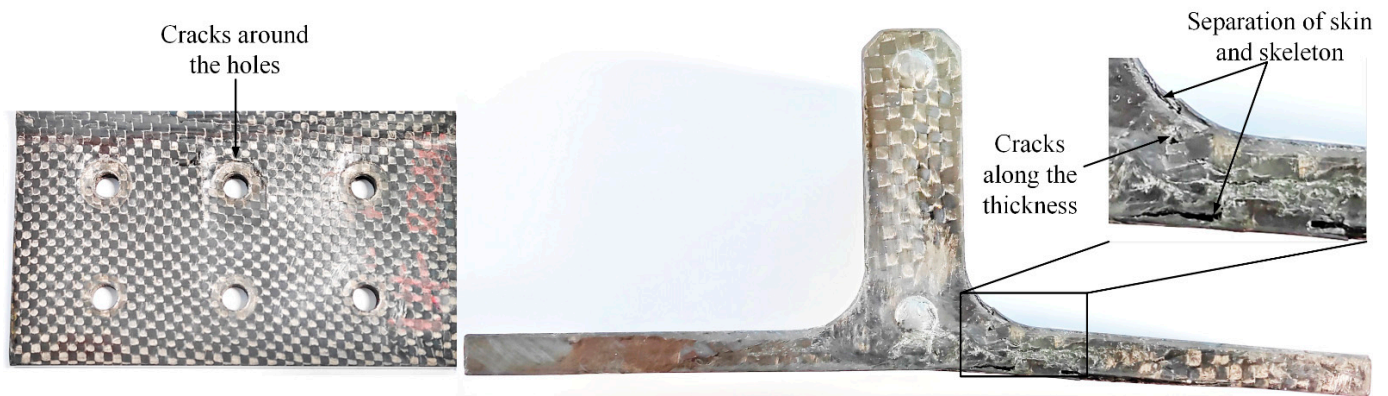
Figure 7. Damage morphologies of the specimen.
