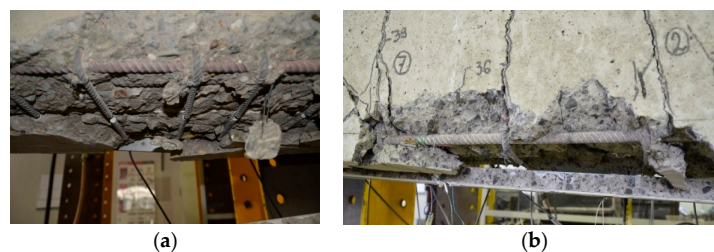
Figure 8. Separation of a large concrete cover in beam B60-214-1T-30 strengthened with 30 mm deep profile: (a) bottom side of beam with cut stirrups after T profile separation; (b) debonding of profile with concrete cover separation.
