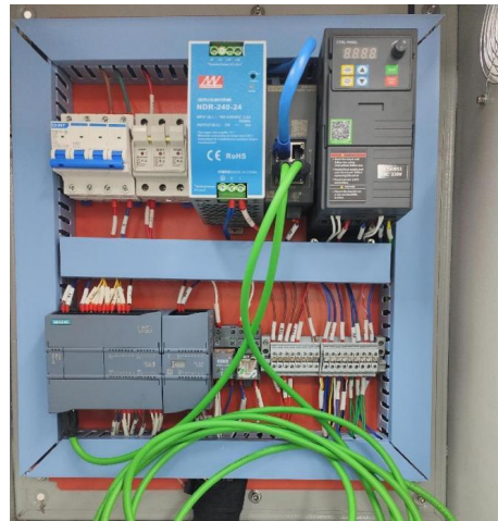
Figure 7. PLC control system.
