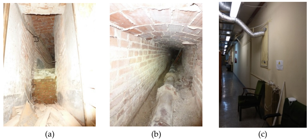
Figure 4. (a) Gallery A, inner space observed from the entry door. (b) Gallery A, back. Inner space observed from Hole 1. (c) Gallery A, corridor, and door with the extraction system.
