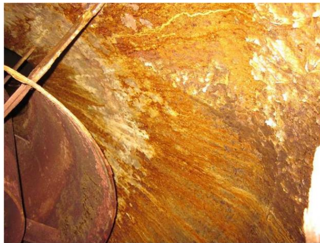
Figure 6. Sulfuric acid corrosion inside the pipeline [28].
