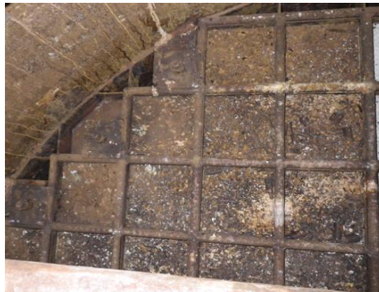
Figure 7. Catalyst blocks clogged by scales of rust [28].
