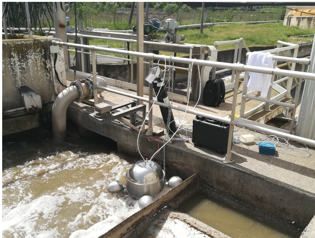
Figure 2. Dynamic flux chamber for the collection of odors in a WWTP (pretreatment). Source: the authors.
