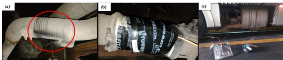
Figure 2. Encapsulation of gases using high-strength aramid tape aided by torofita: (a) Dark color, indicating possible gas leakage; (b) Enclosed location with gases channeled through pipes; (c) Sample collecting container, receiving the channeled cases.
