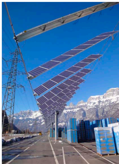
Figure 1. Example of the flexible PV system installation [7].
