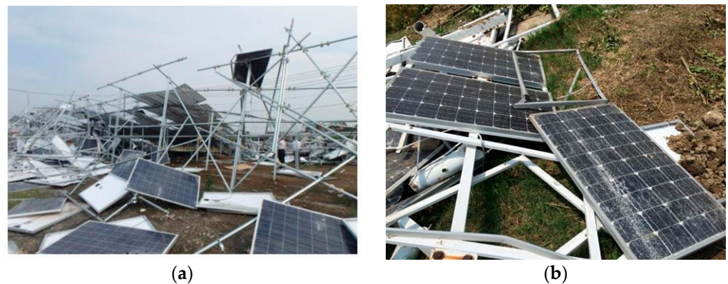
Figure 3. Example of wind-induced damages on PV panel arrays: (a) In Iseisaki city, Gunma prefecture, Japan in 2015; (b) In Yancheng city, Jiangsu province, China in 2015.
