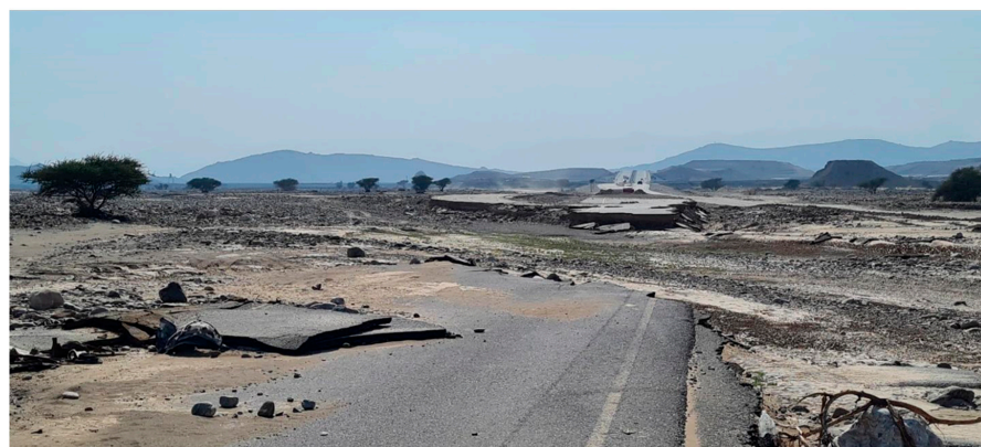
Figure 17. (Top): The flood plain of Wadi Hawasnah one month after the cyclone Shaheen passed as viewed from eastwards. (Bottom): Drainage basin as viewed from downstream/westwards. The wadi bedload deposits destroyed the main road.
